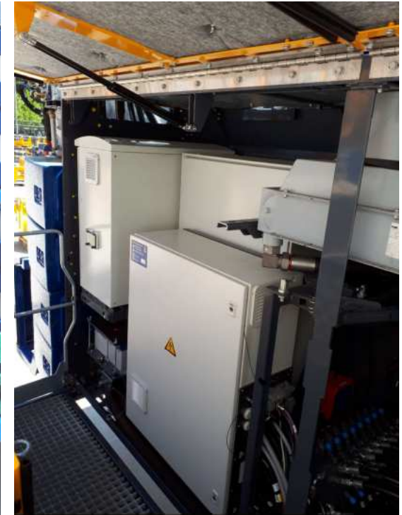
Additional electric cabinets
